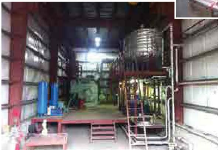
EOS TEXTILE, Bangladesh Daihatsu Diesel generator 6DK-28
