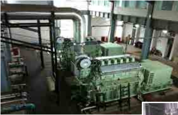
RENATA LIMITED, Bangladesh Pharmaceuticals Company Daihatsu Diesel generator 6DK-26
