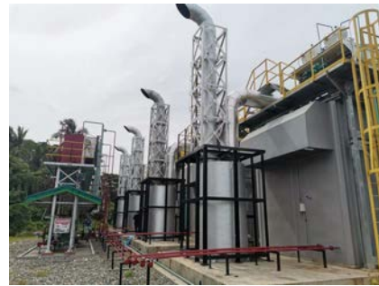
4 x 1.05 MW Containerized Diesel Gensets For BOAC DPP, Marinduque, Philippines
