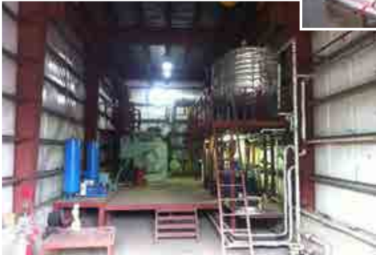
EOS TEXTILE, Bangladesh Daihatsu Diesel generator 6DK-28
